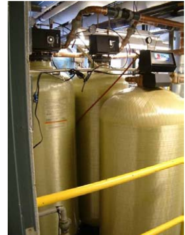
Clarkston, Michigan Arsenic Treatment System installed May, 2003
