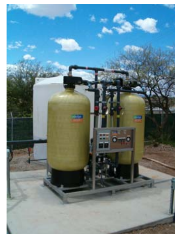
APU-100 System – Rimrock, Arizona Arsenic Treatment Demonstration
